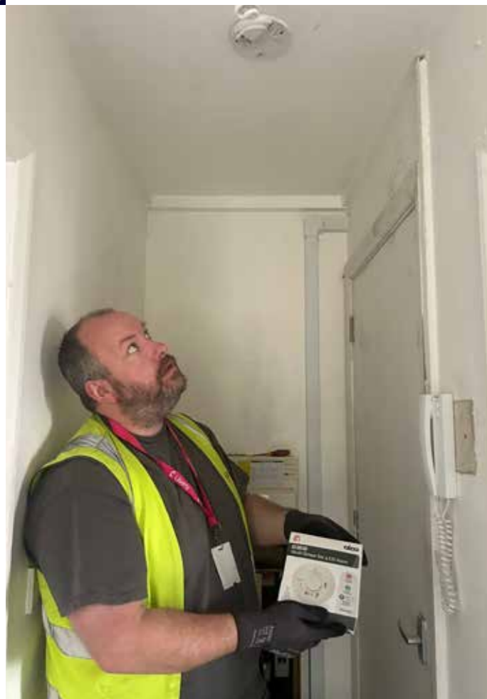
Aico alarms are being fitted to housing for Cheshire West & Chester Council
